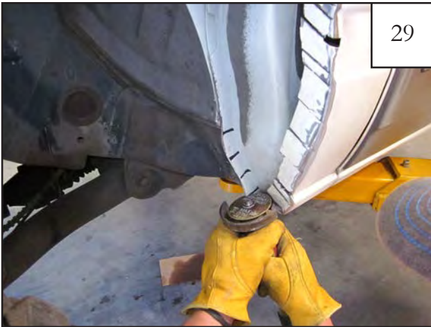
Using a cutoff wheel or other suitable tool, starting at the bottom line, cut horizontal marks in the pinch weld.
