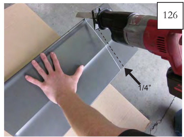
Using a reciprocating saw or other suitable tool, cut the factory side cladding approximately 1/4" back from the line drawn in step 122.
